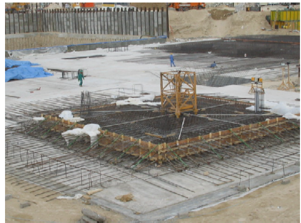
The foundation works for the Wind Tower I's outdoor parking begins to take shape
