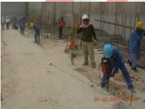
Cathodic Protection Wind Tower I
