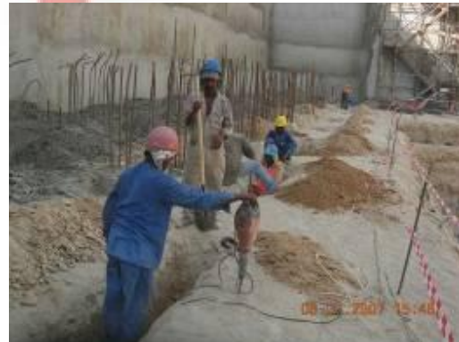
Cathodic Protection Wind Tower I
