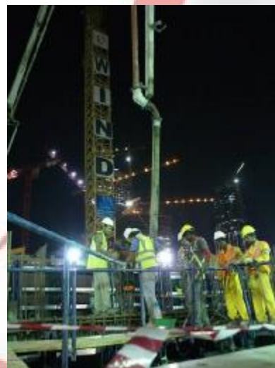
Wind Tower II
