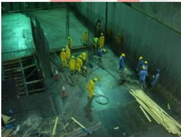
Wind Tower I
